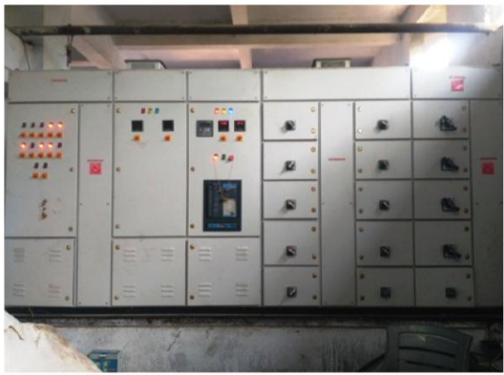
Main Electrical Panel
