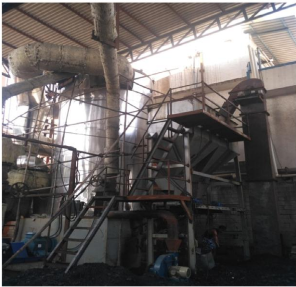
Multi Fuel Fired Boiler
