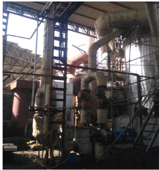
Multi Fuel Fired Boiler
